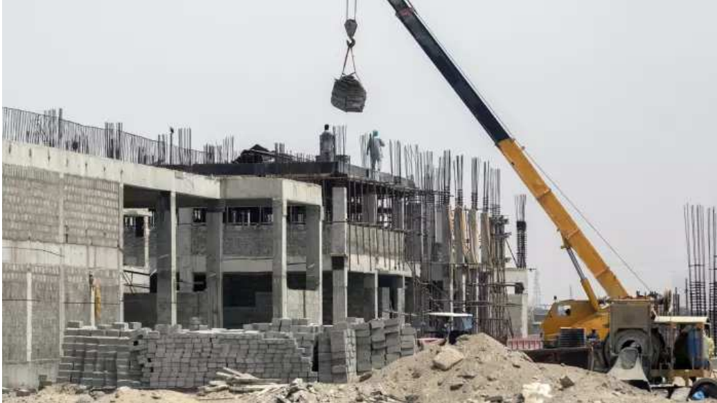
A crane operates at a development site, operated by China Overseas Ports Holding Co, near Gwadar Port in Gwadar, Balochistan, Pakistan © Bloomberg Yu Jie, London School of Economics YESTERDAY
